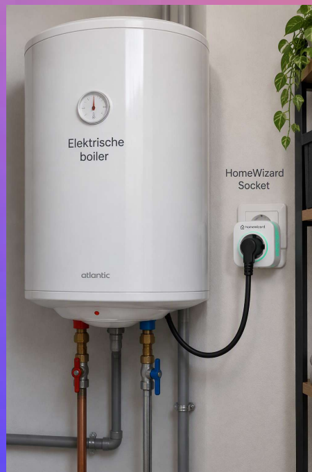
Electrische boiler geschakeld via Homewizard i.c.m. combi Cv-ketel
